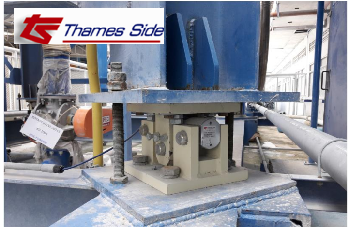
PVC & CaCo 3 , Silos weight monitoring system
